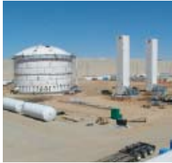
THE 1.8-MILLION-GALLON STORAGE TANK NEARS COMPLETION IN MARCH 2007 AT THE NEW CLEAN ENERGY CALIFORNIA LNG PLANT IN THE MOJAVE DESERT.
