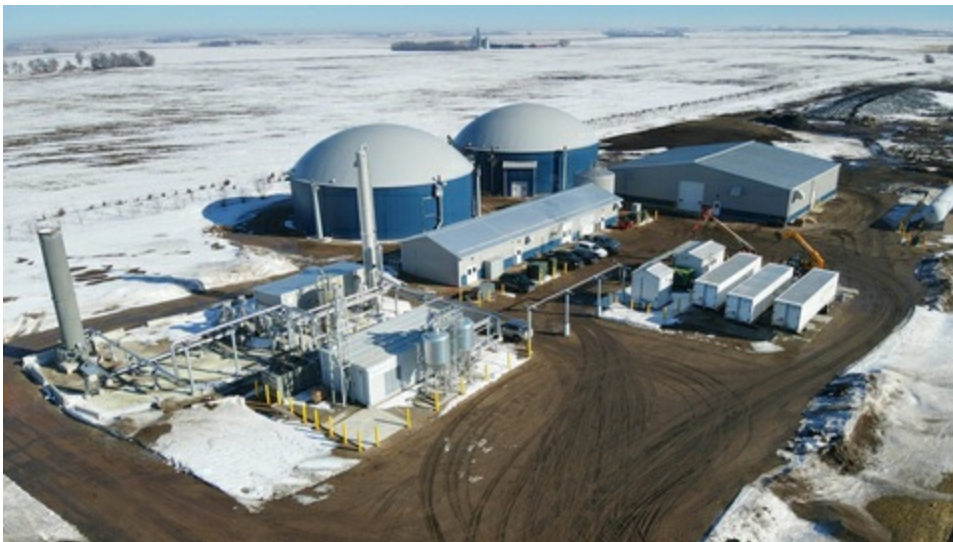
Tri-Cross Dairy Clean Energy RNG (renewable natural gas) digesters and production facility (Photo: Business Wire)
